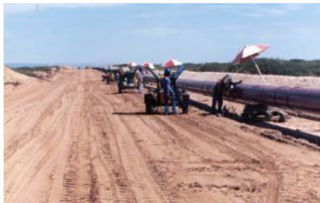
Figure 2-2: Transmission Pipeline in the Americas (Hopkins, 2002)
