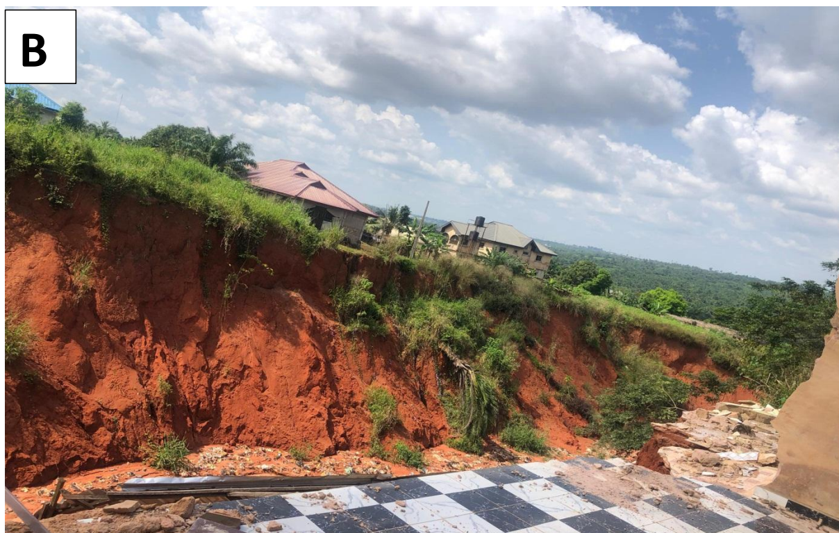
Plate 3.1 A and B: Gully erosion site in Evbhomore community in Ovia North East Local Government Area of Edo State
