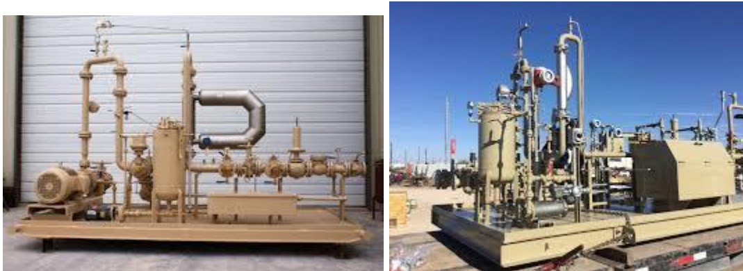
Figure 1.1.1 : Representative LACT system components (pump, BS&W probe, air eliminator, sampler, meter, prover, valves) as described by industry source,(Image credit: KROHNE/Angus Measurement)
