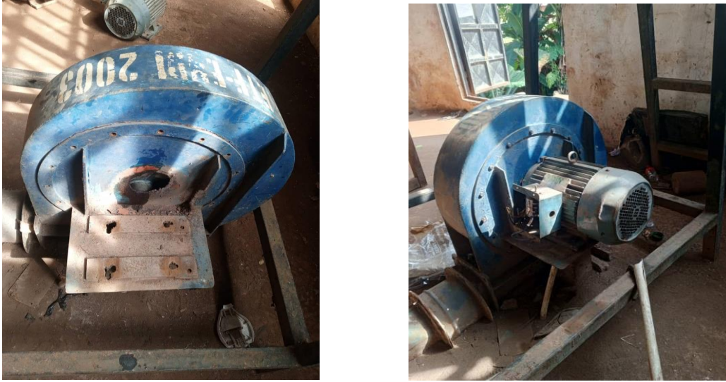
Figure 4.2: Maintenance of Drive Motors and Mechanical System
