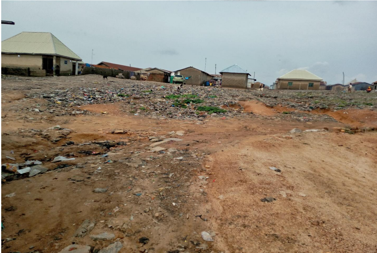
Plate 6.4: Poor quality road at Anagada Satellite Town Source: Data from field survey
