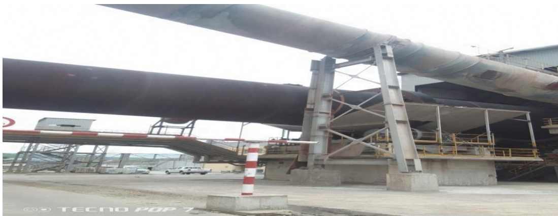
Figure 2.6b Cement Rotary Kiln.( Bua Cement Plant, 2025)
