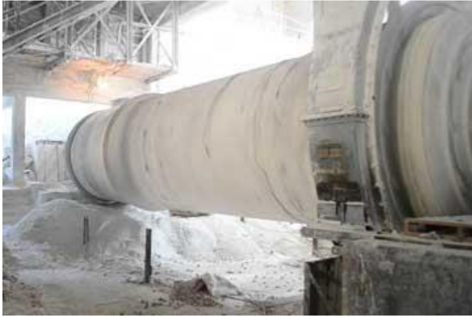
Figure 2.7: Cement grinding mill ;( Bua cement 2025)
