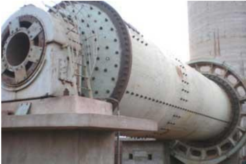
Figure 2.4. Raw mill; ( Bua Cement plant, 2025 )
