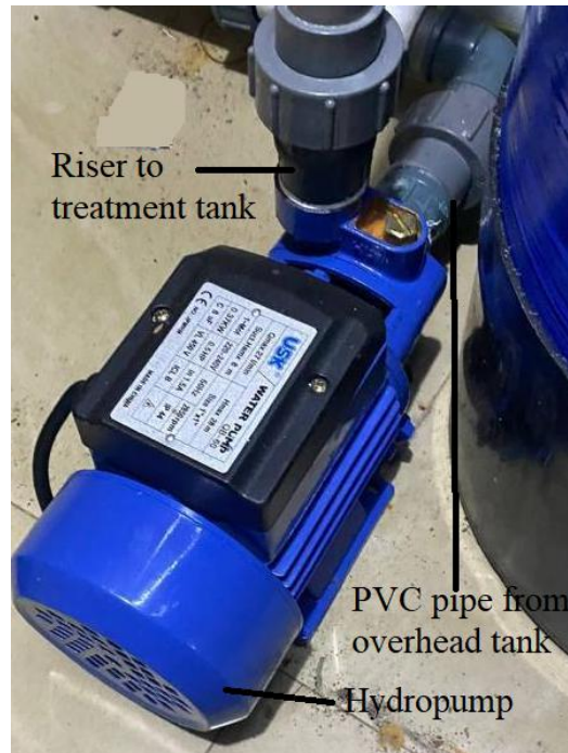
Figure 3.3 Hydro-pump and interconnections
