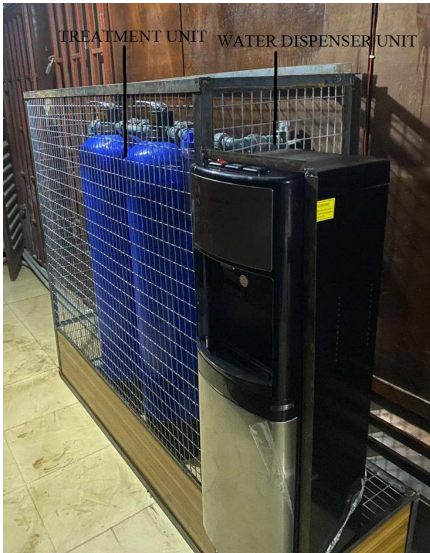
Figure 3.6 The Fabricated Water Treatment and Dispensing Facility at the Production Engineering Department Annex
