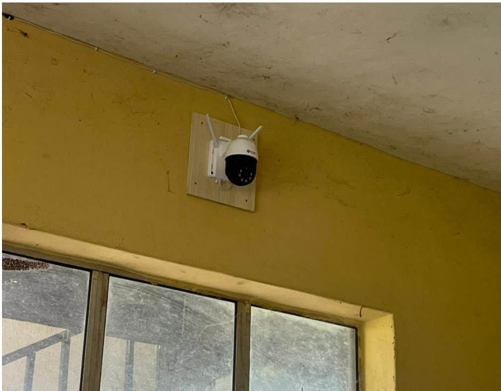
Figure 7 - Solar Camera Mounted on Classroom Wall
