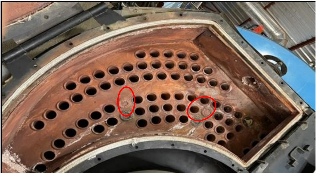
Figure 4.1: Blocked boiler tubes in the third pass.
