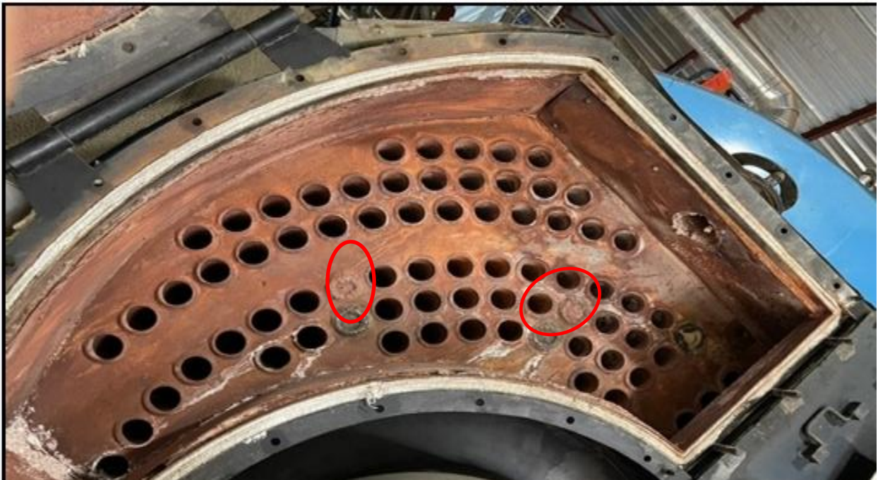
Figure 4.1: Blocked boiler tubes in the third pass.
