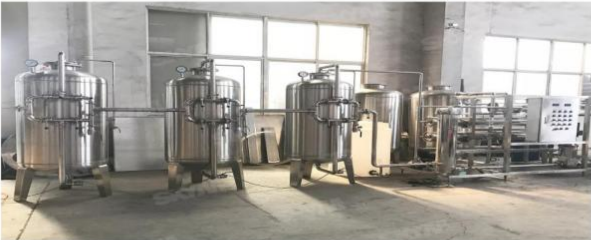
Figure 2.17: A Three Tank Water Filter
