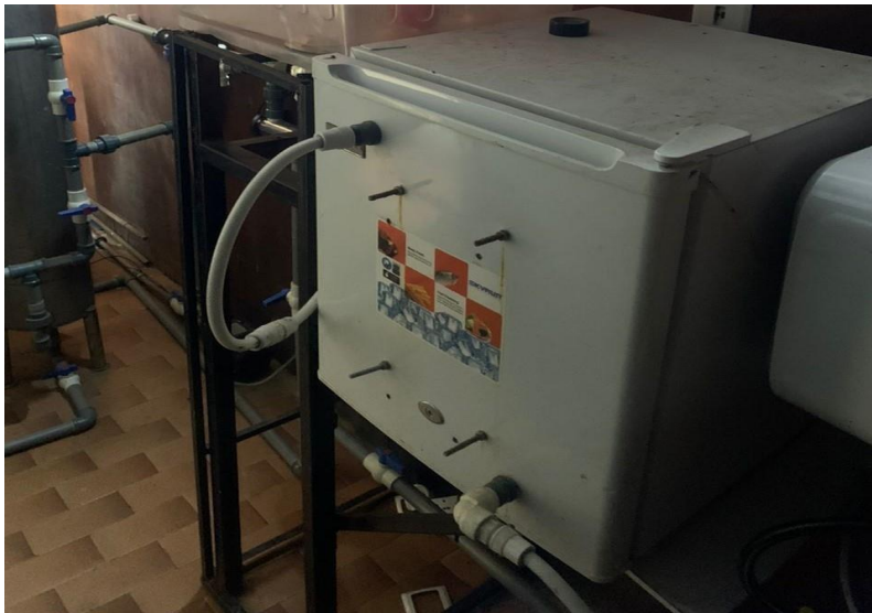
Figure 3.6: Refrigerator and Heater Stations
