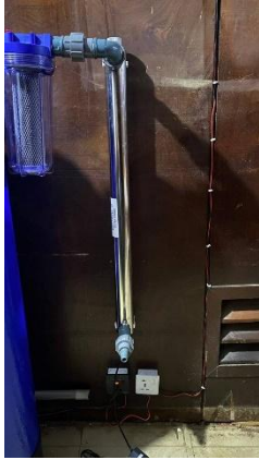
Figure 3.3: UV Treatment set-up
