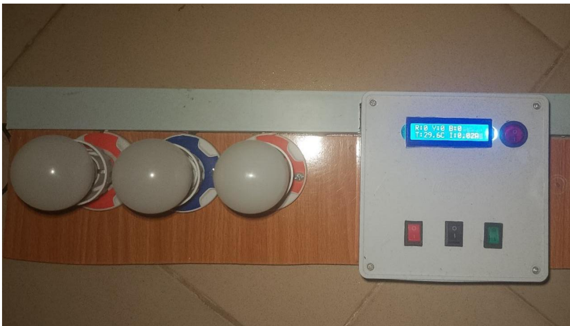
Figure 4.9 Faulty Operating Condition Due To Under Voltage Of Three Phases
