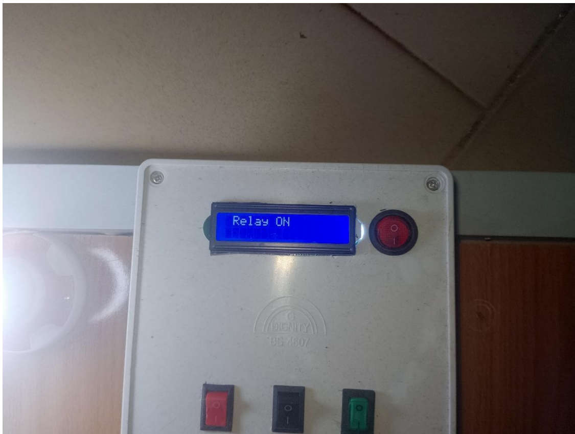
Figure 4.14 Three Phase Induction Motor Protection System Restored To Normal Operating Condition(Closer View)
