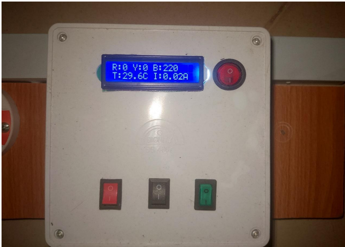
Figure 4.10 Faulty Operating Condition Due To Under-Voltage Of Two Phases
