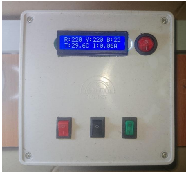
Figure 4.5 Three-Phase Induction Motor Protection System in Normal Operating Condition Closer View (Complete System)
