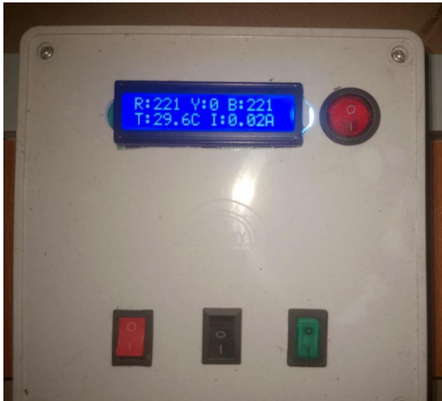
Figure 4.11 Faulty Operating Condition Due To Under-Voltage Of One Phase
