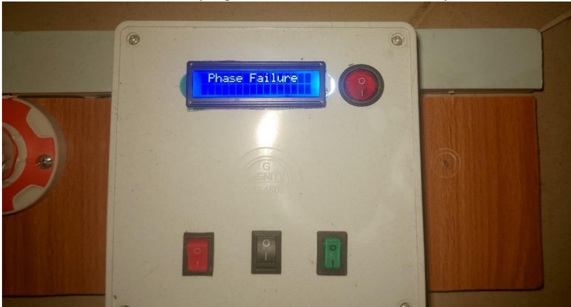
Figure 4.8 Faulty Operating Condition
