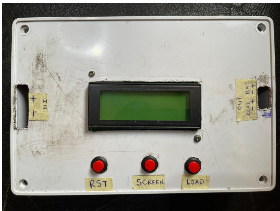
Figure 20: The Protective Cover of The Charge Controller
