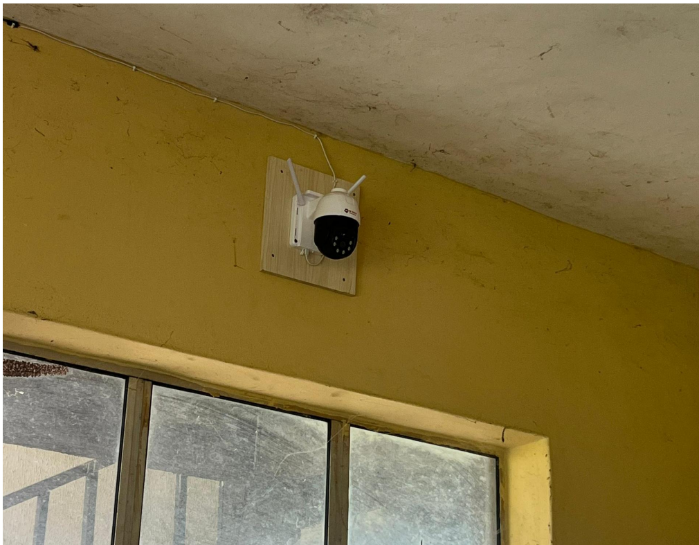
Figure 7 - Solar Camera Mounted on Classroom Wall
