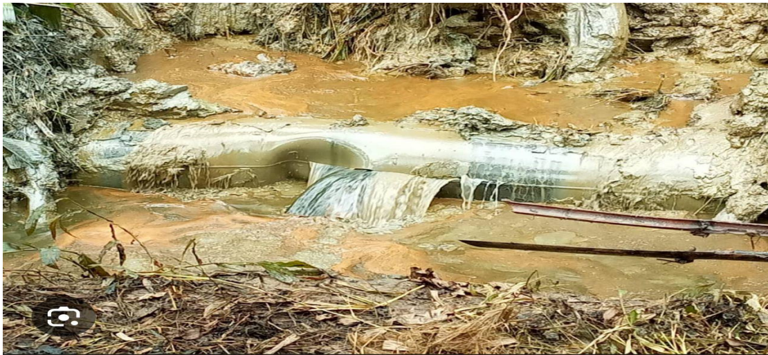
Fig8: Ruptured spot on the Ogodu-Brass Pipeline oil spill which is the fourth oil spill recorded from Agip's Ogodu/Brss Pipeline 41
