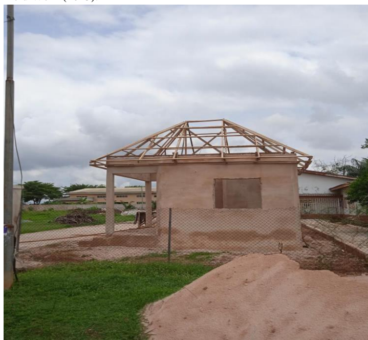
Plate 2: Side view of the pitched timber roof framework under construction Source: Researcher Field Work (2025).
