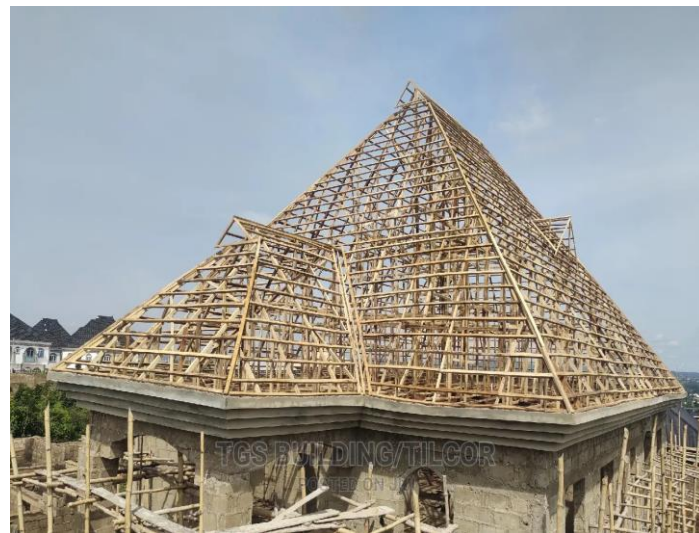
Plate 1: Overall view of the timber roofing structure nearing completion Source: Researcher Field Work (2025).
