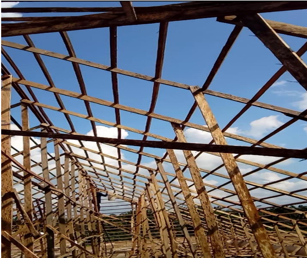
Plate 3: Ongoing construction showing multiple timber trusses in place Sources: Researcher Field Work (2025).
