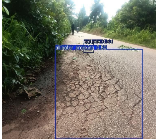
Fig 4.19: Alligator Crack detected with 80%
