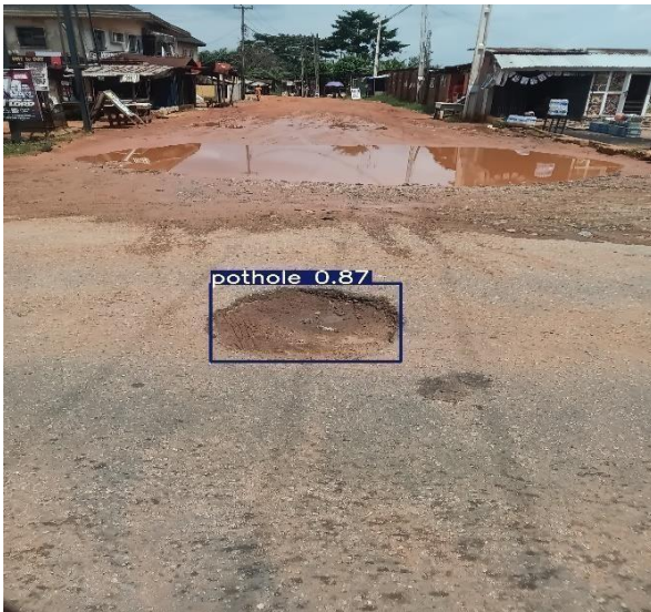
Fig 4.17: Pothole detected with a precision Level of 87%
