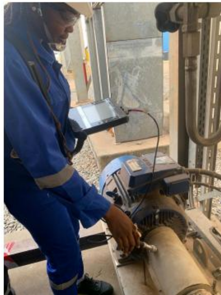
.Figure 2.1: A Centrifugal Pump [Azura Power Plant]
