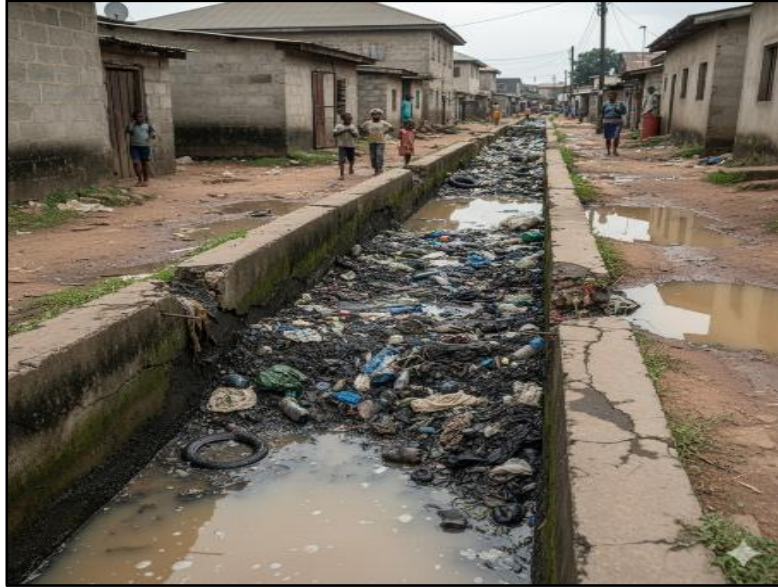
Figure 2.5: Example of severe sediment and debris accumulation compromising the flow capacity of an urban drainage channel.
