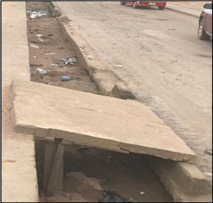
Figure 4.2: Structural failure characterized by a displaced concrete cover, indicating differential settlement and a critical safety hazard along the drainage alignment.
