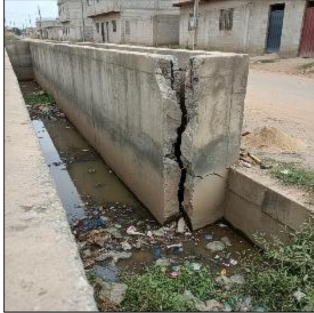
Figure 2.1: Common structural failure (cracking in a rectangular concrete drainage channel).
