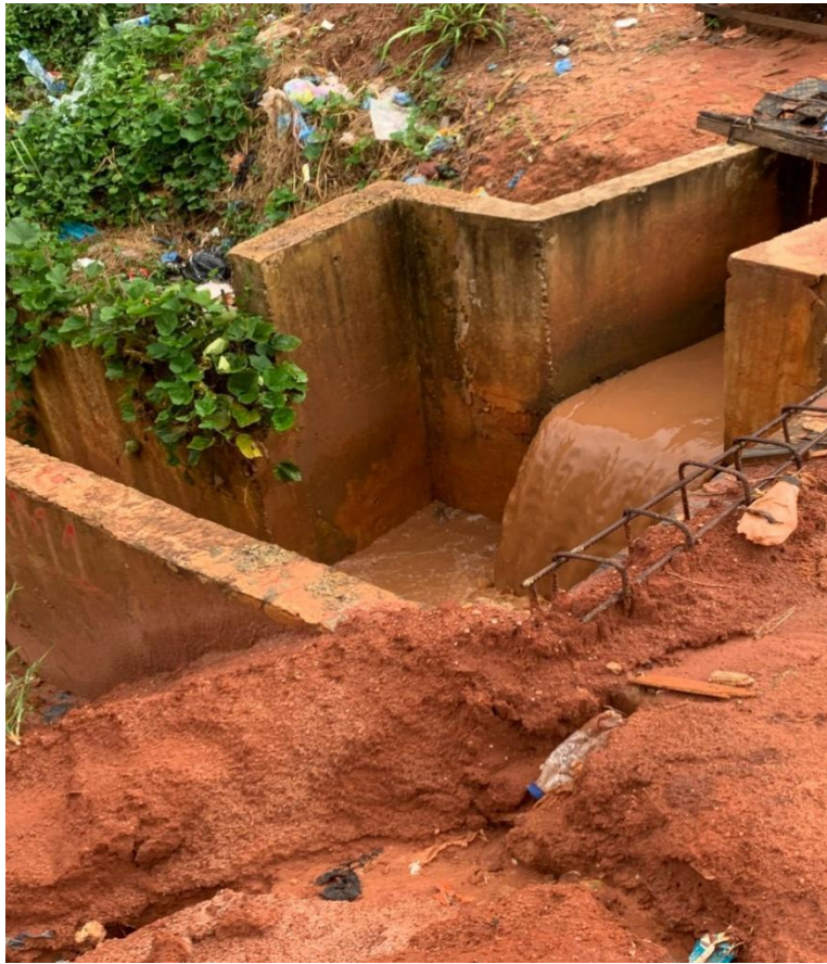
Plate 3.3: Dumping of refuse in drainage canal in Amufi community
