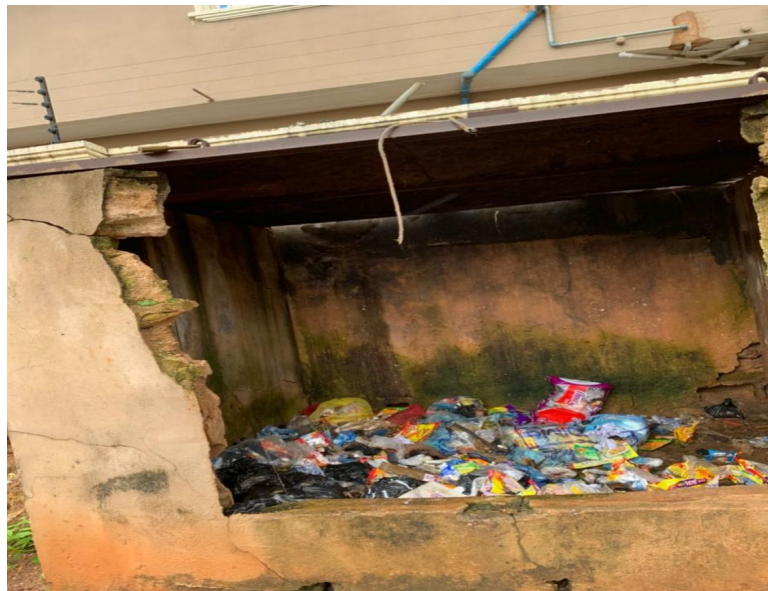
Plate 3.2: Dumpsite in Amufi community
