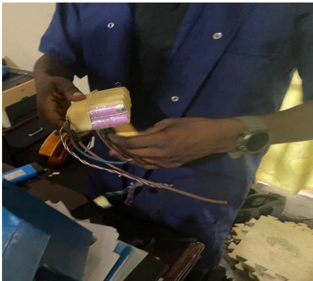
Figure 3.2: The Batteries been arranged
