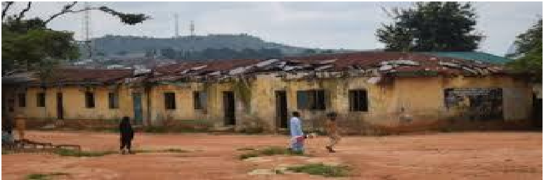
Figure 1: A dilapidated secondary school building in Ovia North East local government area of Edo State
