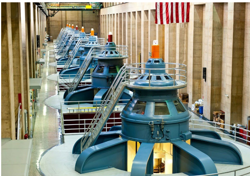
Fig 2.2: Hydroelectric Power Generator
