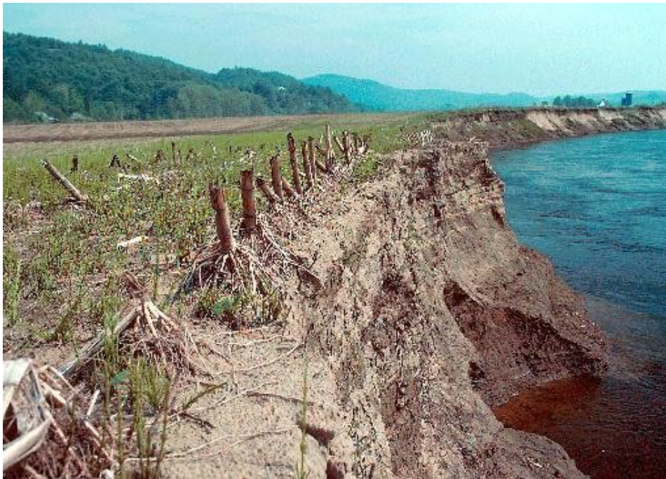
Fig. 2.4: Scouring of River Banks
