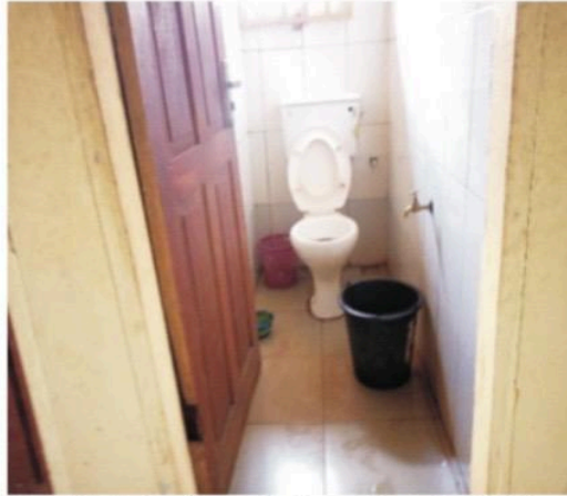
Plate 2: Flush toilet at Uselu market toilet facility
