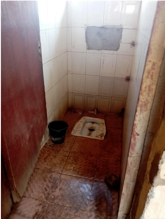
Figure 2.2: Toilet stalls condition of Aoma market, Uzzeba, Owan west
