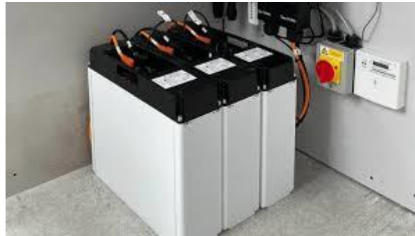
Figure 2.6: Lead Acid Batteries
