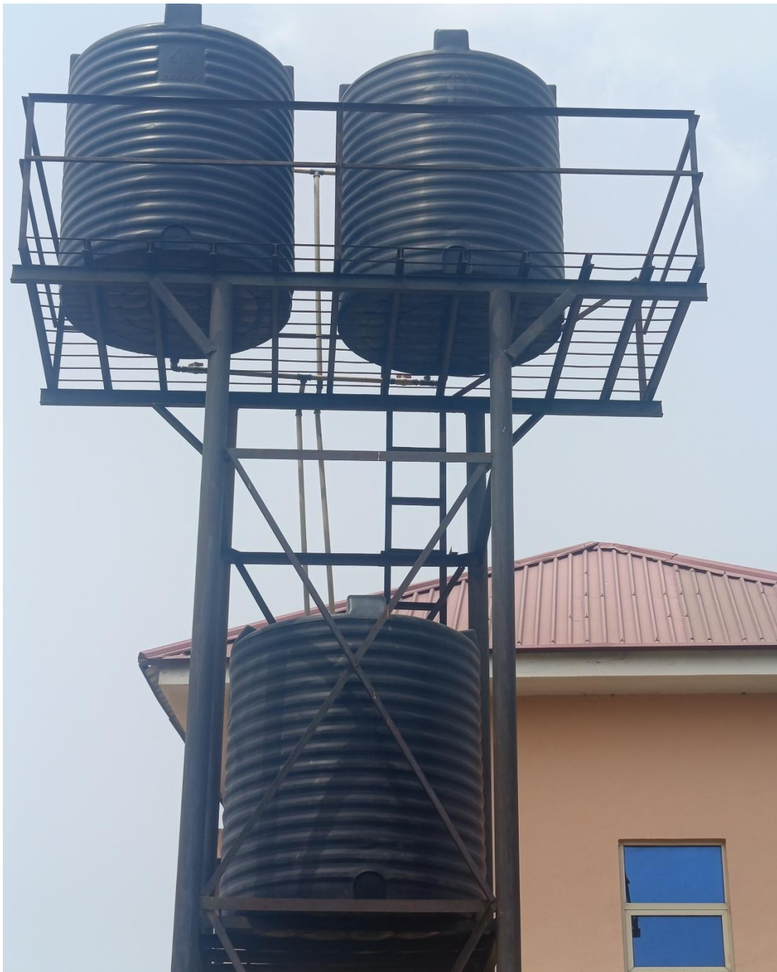
PLATE D-1. A Storage tank
