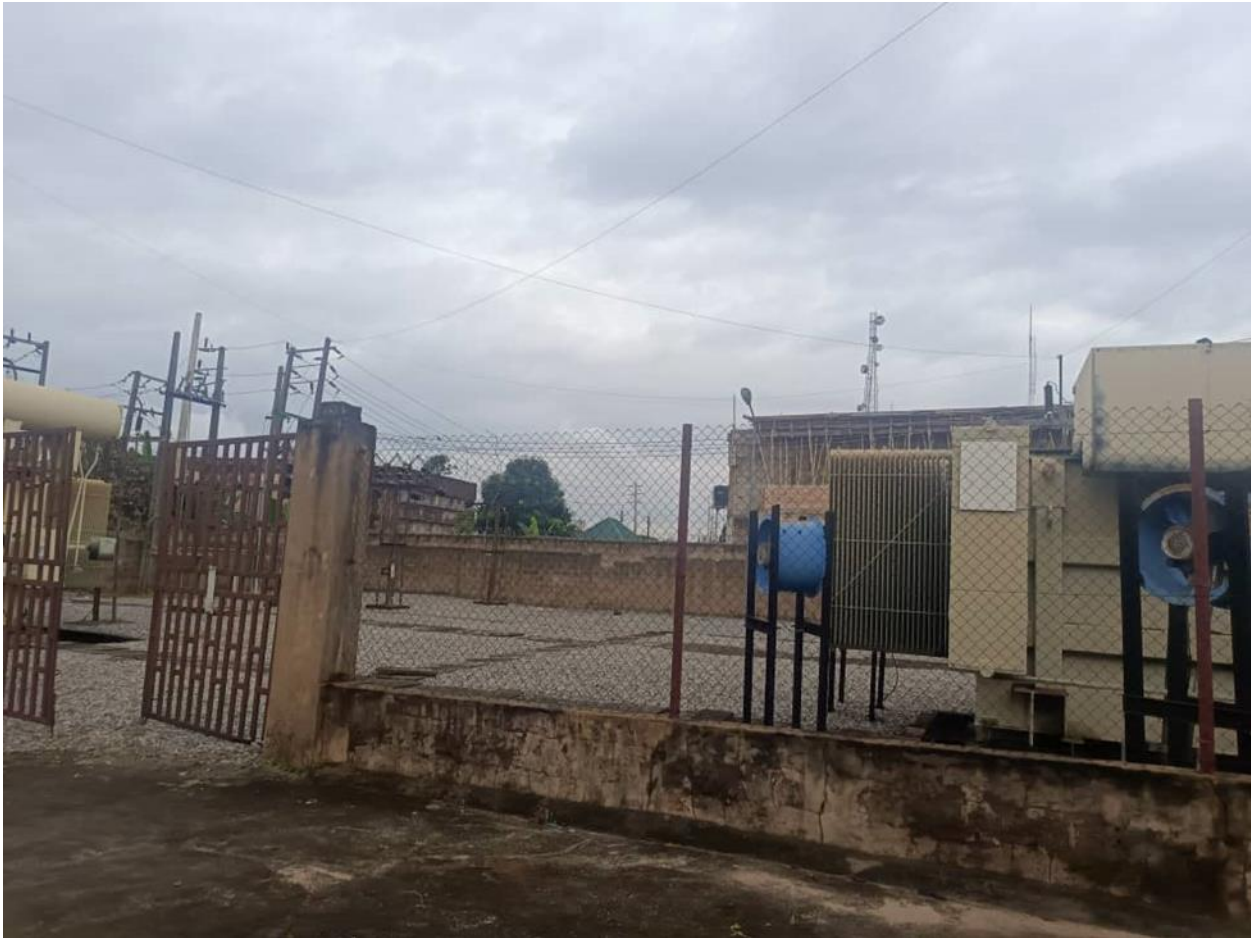
Fig 2.1: Picture showing the GRA 33/11kV Injection Substation
