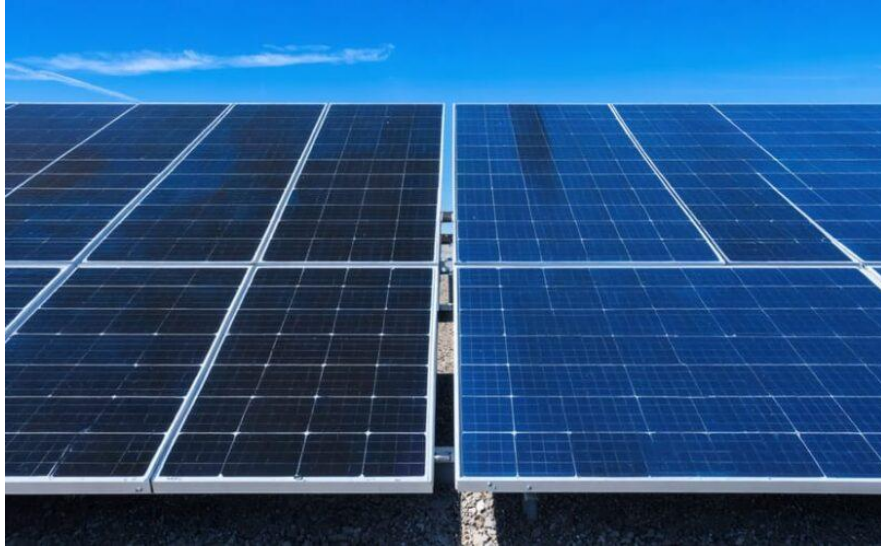
Figure 2.2: Monocrystalline Solar Panels
