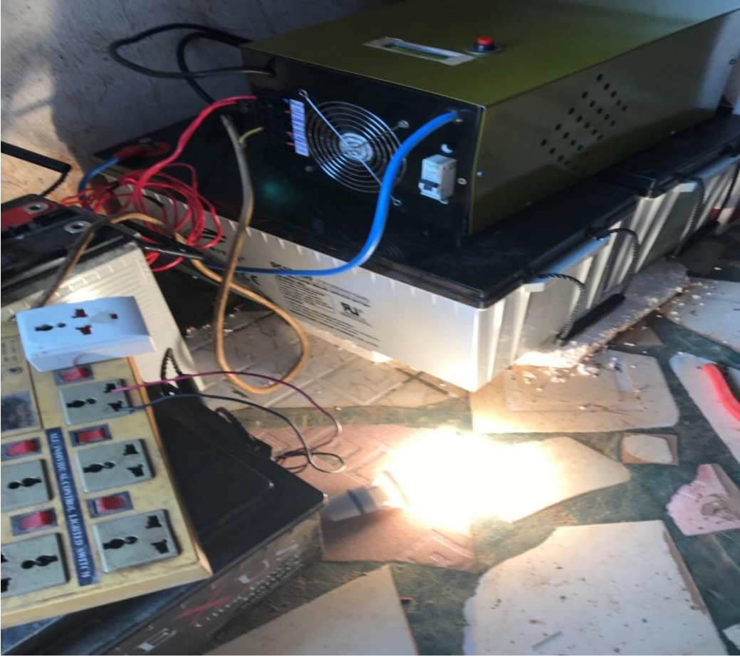
Fig 4.11: the 2KVA inverter on load test
