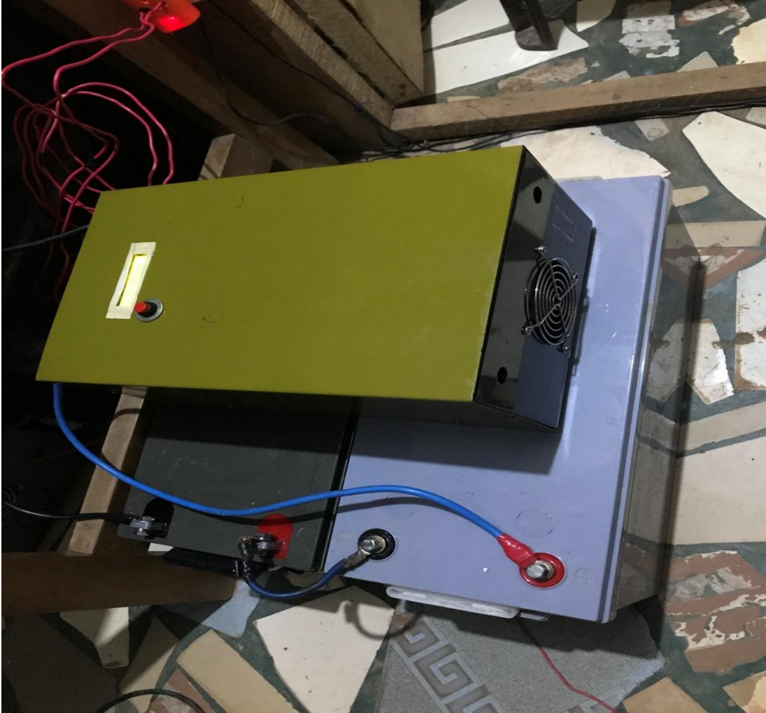
Fig 4.12: the 2KVA inverter connected to mains to charge the batteries
