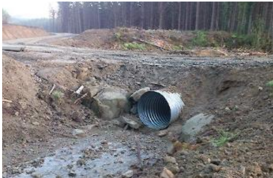
Figure 2.5: Progressive deterioration of culvert outlet due to foundation scour (Source: NZ Forest Road Engineering Manual, 2012)
