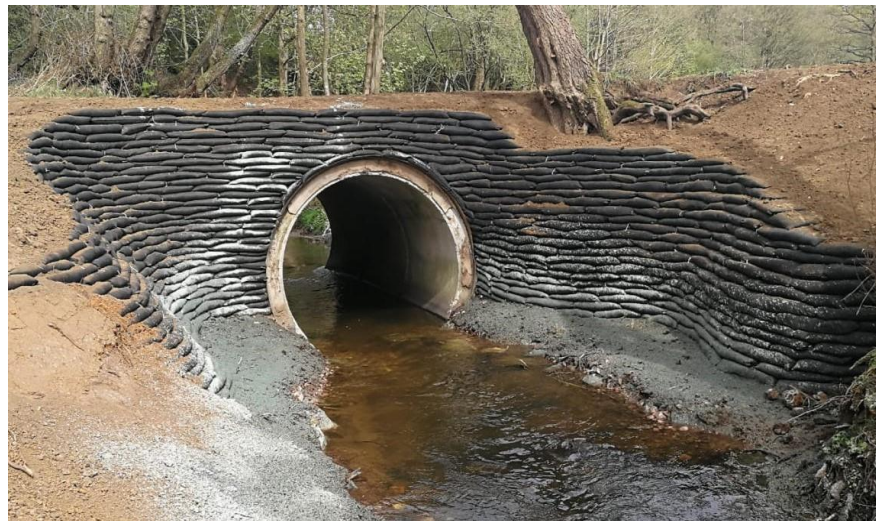
Figure 2.2: Circular concrete culvert in operation during a storm flow event (Source: Atlantic Industries Ltd, 2023)
