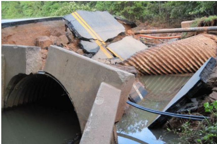
Figure 2.6: A damaged box culvert showing the effects of structural distress (Source: Tenbusch Inc., 2013)
