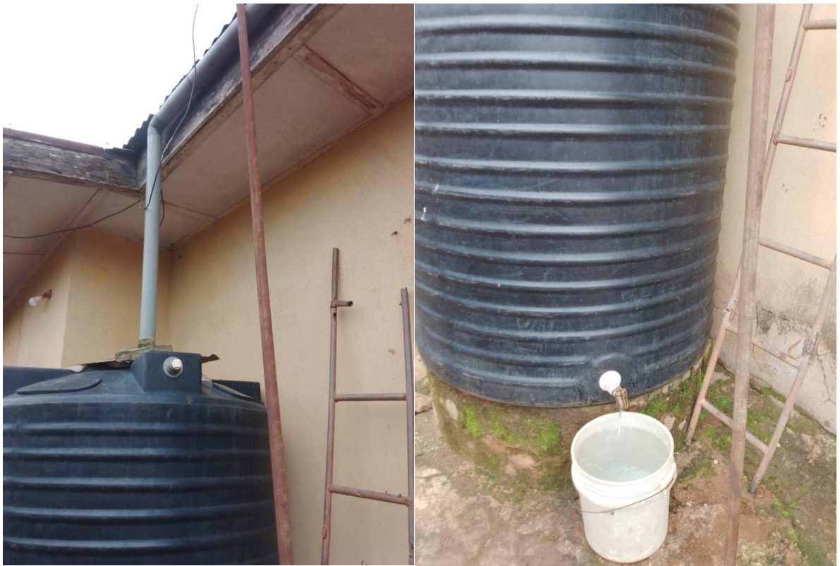
Fig. 4.2 Rainwater harvesting system observed in Eyean, Benin City.
