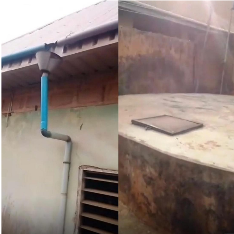
Fig. 4.1 Rainwater harvesting system observed in Upper Sakponba, Benin City. The left image shows a locally fabricated funnel and PVC pipe assembly attached to the roof gutter, designed to channel rainwater downward. The right image shows the receiving concrete well (5,000 litres of water storage capacity), where harvested water is collected for various domestic uses.
