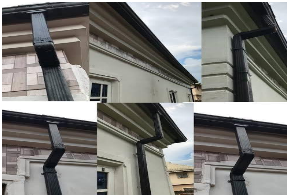
Fig. 4.3 Modern rainwater harvesting system at a residential building in Amagba Road.
