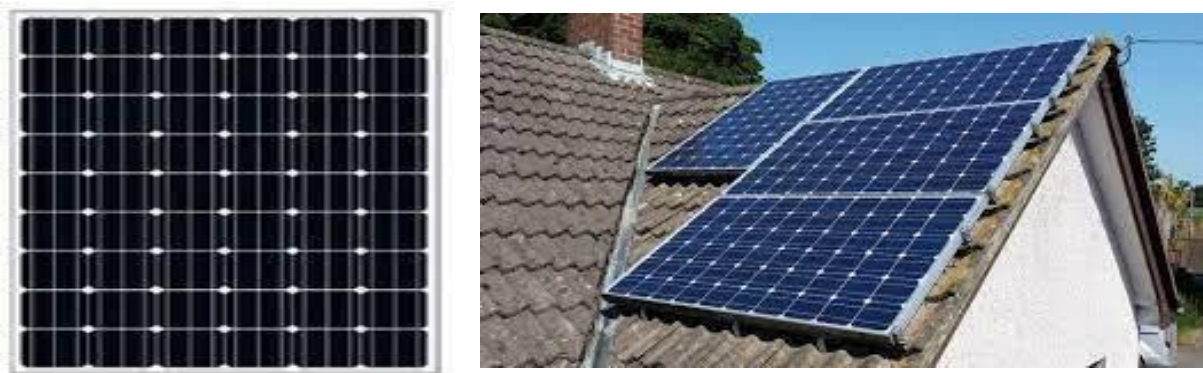
Fig 2.2: Solar Panel Mounted On A Rooftop
