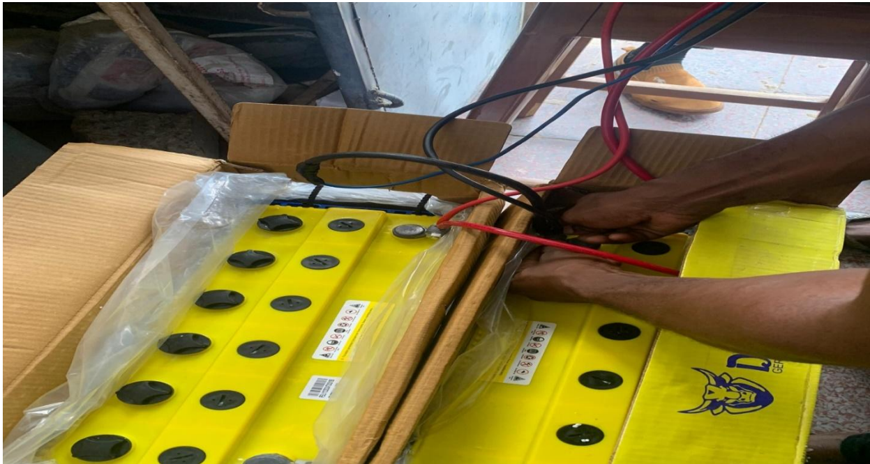
Fig 5.3: Two 12V batteries being connected in series
