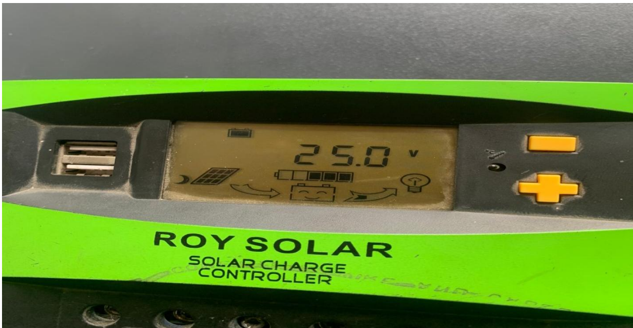
Fig 5.6: A charge controller showing the battery voltage
