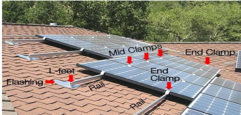
Figure3.1.3 image of Solar Panel Rails
