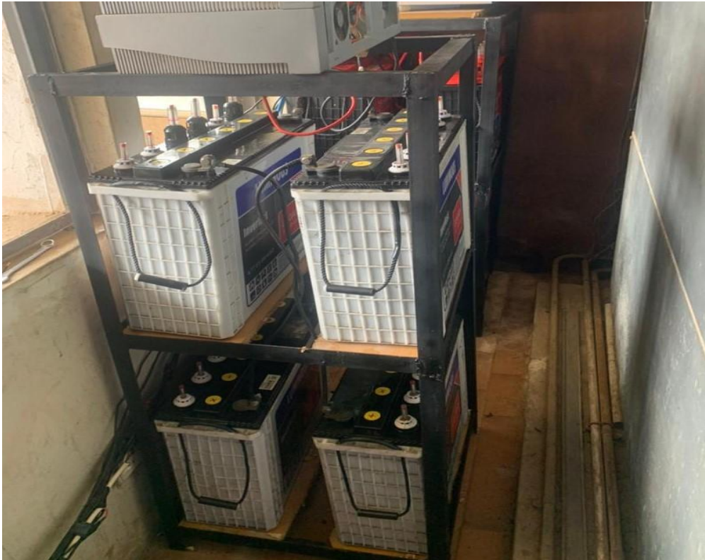
Fig 7: showing the arrangement of batteries in frame
