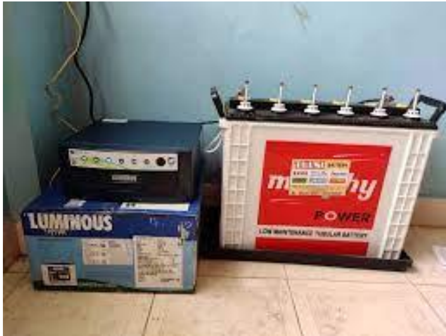
Figure 24: Interconnection between Solar Panels, Battery, and Inverter
