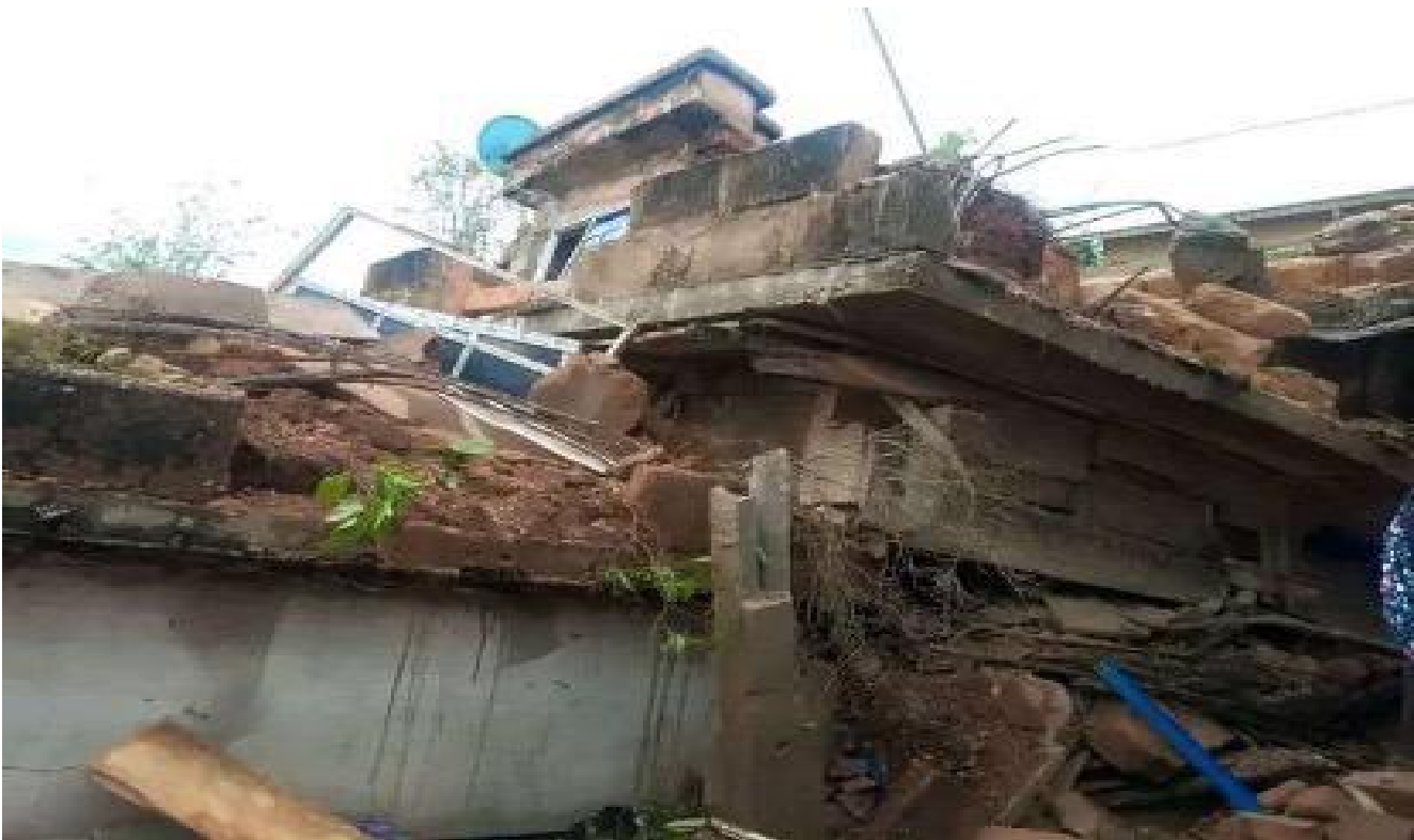
Plate D - 3: Building after collapse
