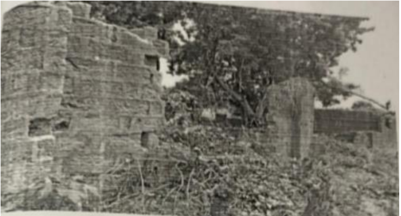
Plate E- 3: Building after collapse
