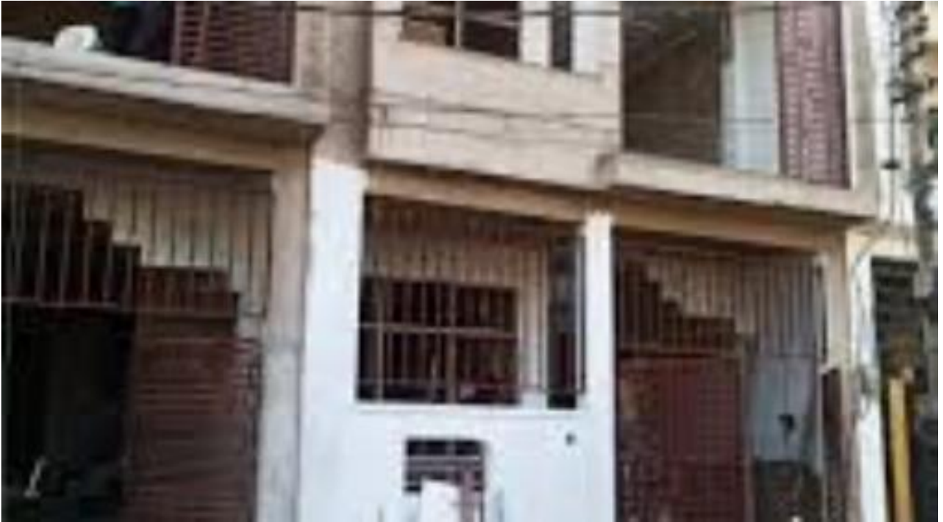
Plate C - 2: Building before collapse
