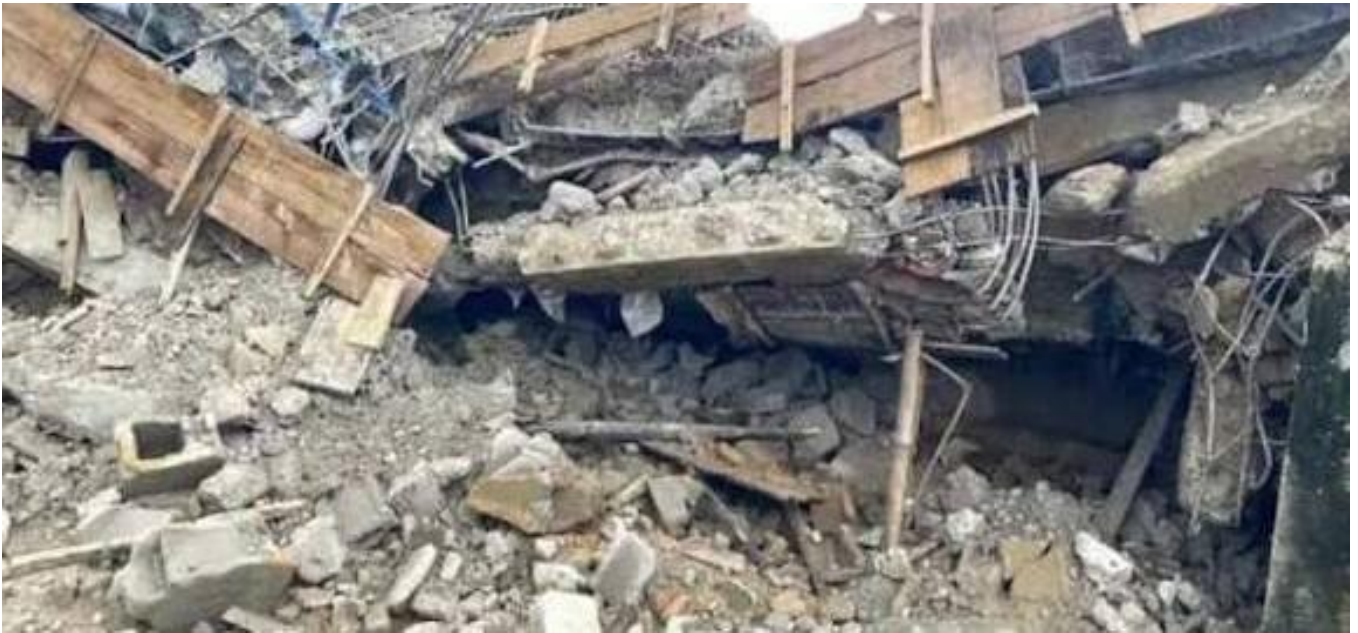
Plate C - 3: Building after Collapse
