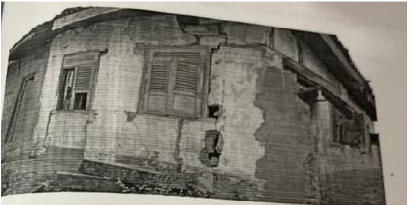
Plate B - 2: Building after collapse
