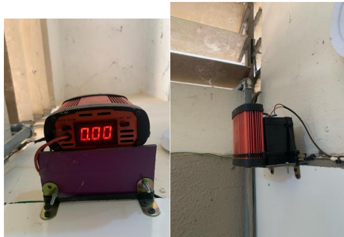
Figure 3.6 DC Battery Charger
