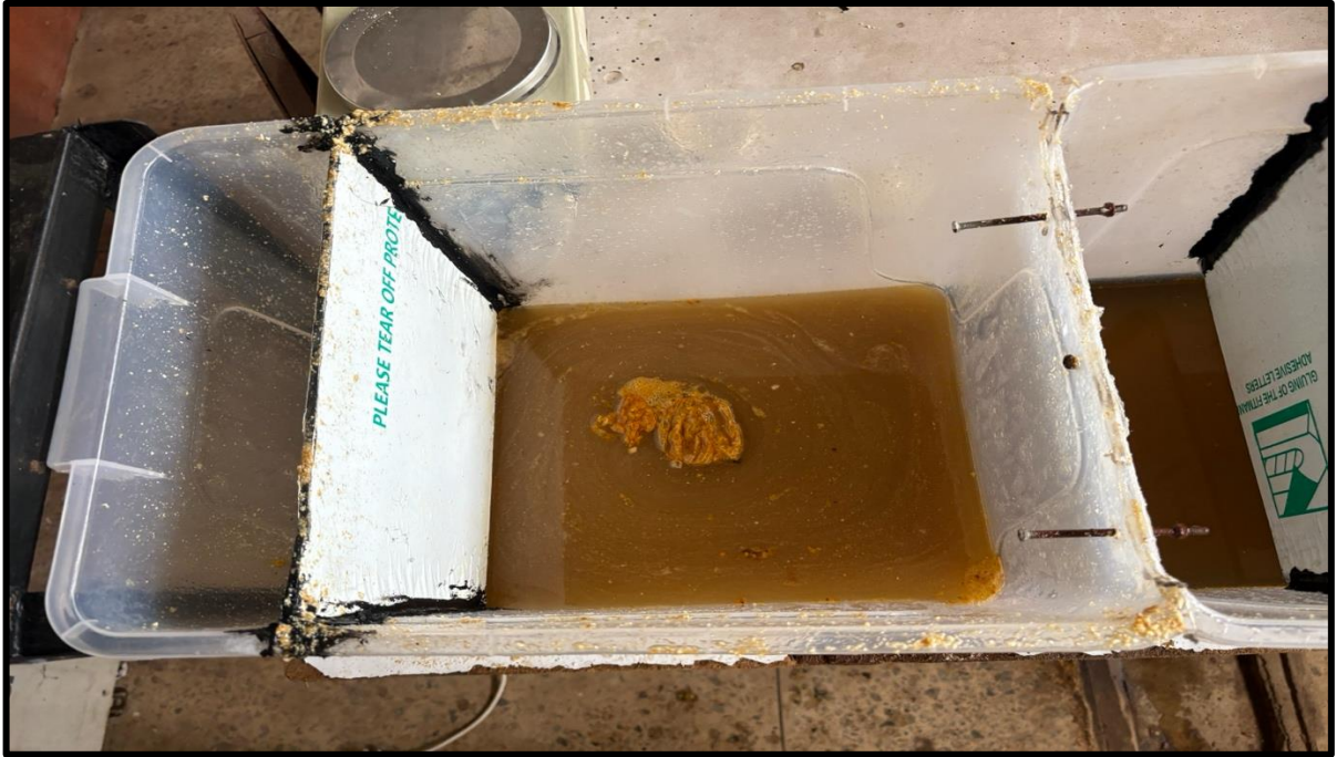
Plate 3: Greywater in the Coagulation Basin of the Facility
