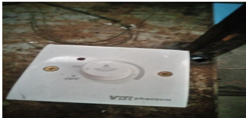
Fig 3. 38 Showing variable speed controller
