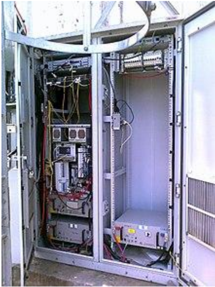
Fig 2.1: Electronic equipment box at the base of cellphone tower.
