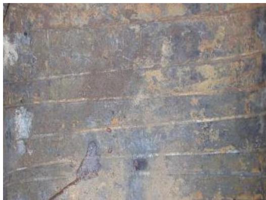
Specimen 1a (Above ground) External metal surface underneath Tape coating
