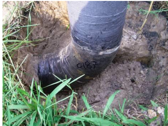
Figure 3.4 shows Pipeline 4 segment from which specimen 4a & 4b were taken
