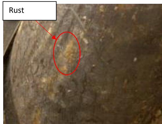
Specimen 2b (Below ground) External metal surface underneath Tape coating
