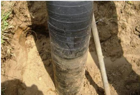
Figure 3.3 shows Pipeline 3 segment from which specimen 3a & 3b were taken
