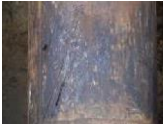
Specimen 2a (Above ground) External metal surface underneath Tape coating
