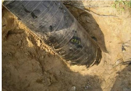
Figure 3.2 shows Pipeline 2 segment from which specimen 2a & 2b were taken
