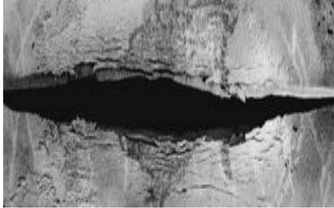
Figure 2.8: Example of colony of stress-corrosion cracks on external surface of high-pressure gas transmission pipeline. The top scale is inches and the bottom in centimeters. (Beavers et al., 2006)
