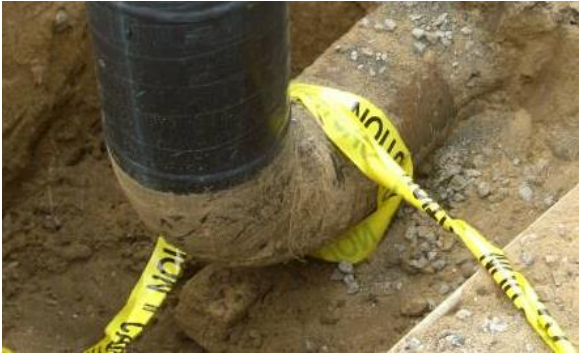
Figure 3.1 shows Pipeline 1 segment from which specimen 1a & 1b were taken
