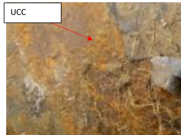
Specimen 4b (Below ground) External metal surface underneath Tape coating
