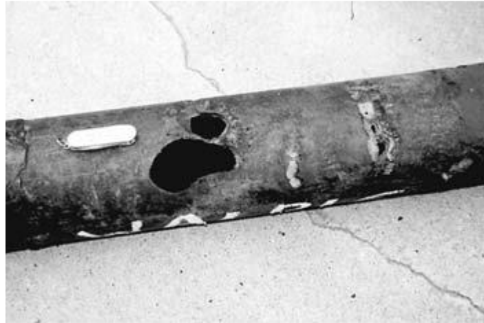
Figure 2.7: Pipeline that experienced stray current corrosion caused by inverting the electrical leads to a cathodic protection rectifier (Beavers et al., 2006)
