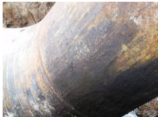
Specimen 1b (Below ground) External metal surface underneath Tape coating
