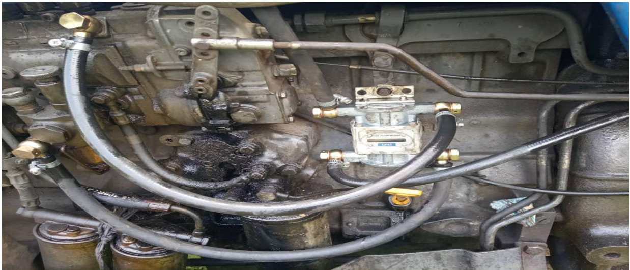
Plate 3.10: Mounting of Fuel Flow Meter
