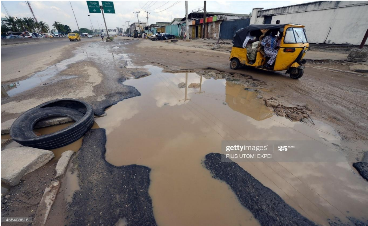
Fig.4.5.7: Potholes infested Apapa-Oshodi Expressway Source: Google Images, 2020.
