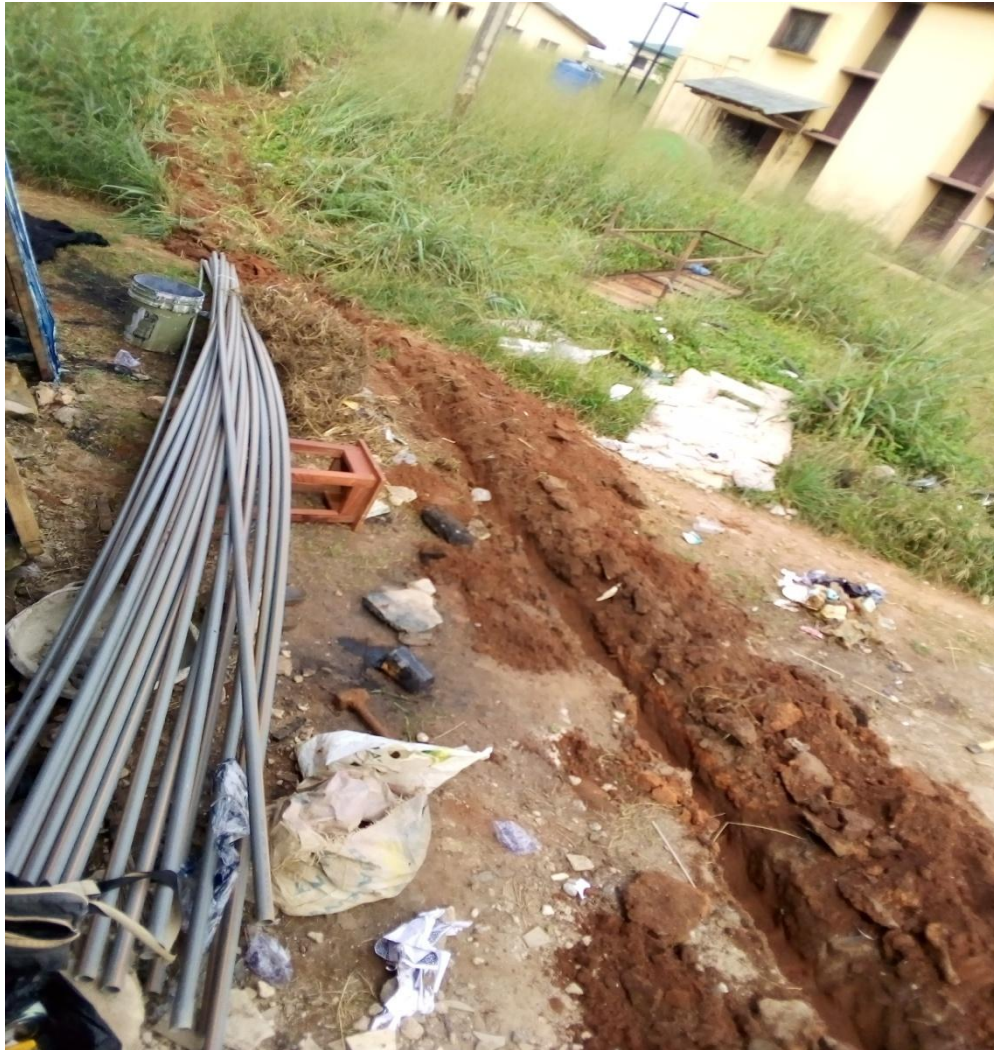
Fig. 9a: Digging of the Ground to Insert the Plumbing Pipes for the Borehole
