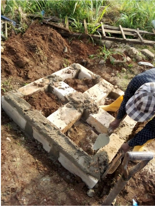
Fig. 10a: Construction of base for Placing of Tank for Borehole Photo Credit: Oyedele Joshua
