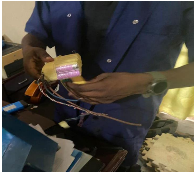
Figure 3.2: The Batteries been arranged
