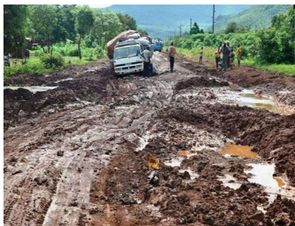
Figure 4.35: Bad rural road with trucks carrying agricultural produce, highlighting transportation difficulties that contribute to post-harvest losses (Source: Pinterest, 2023).
