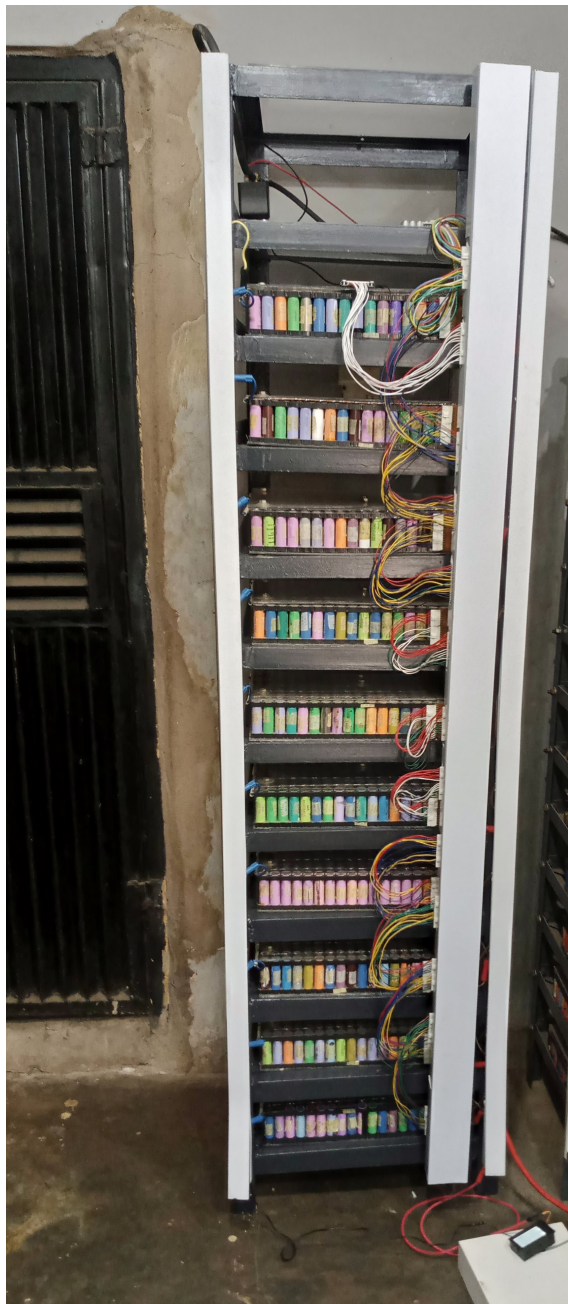
Figure 3.12: Full 10kWh Setup with Rack
