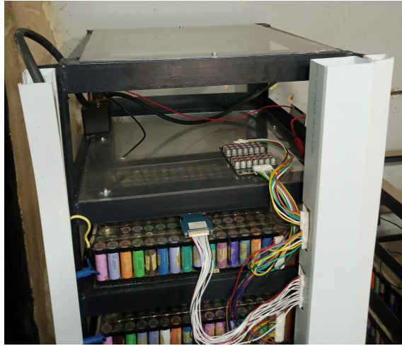
Figure 3.11: Pack showing the BMS, Balancer and Protection Relay
