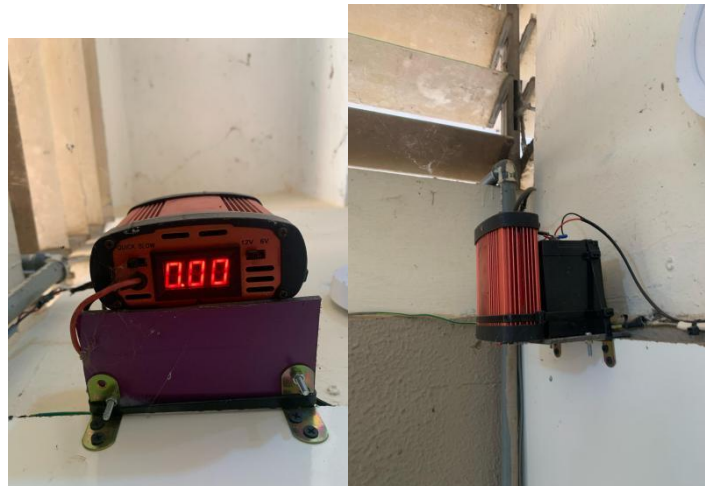
Figure 3.6 DC Battery Charger
