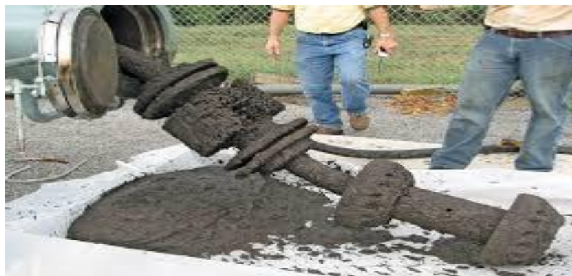
Fig 2.2: Pig launcher at the downstream of a pipe section with some sand after a pigging operation
