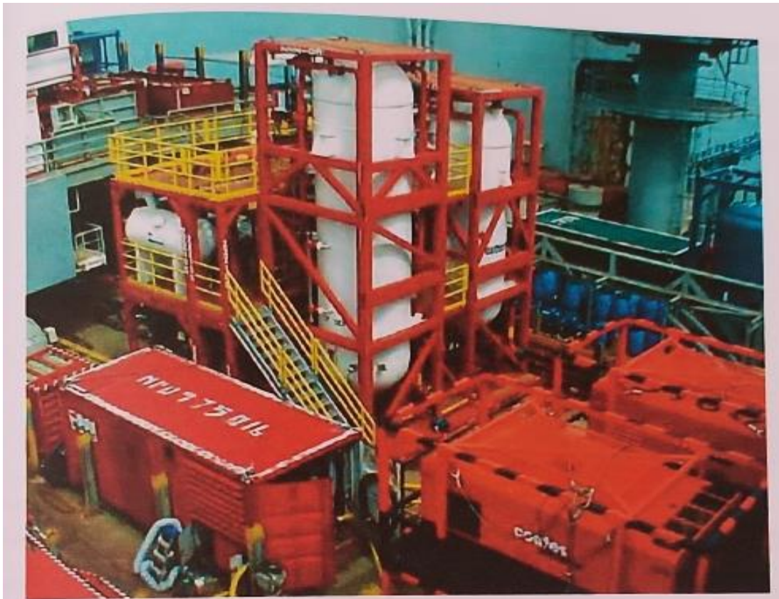
Figure 3.4: Three-phase separation device
